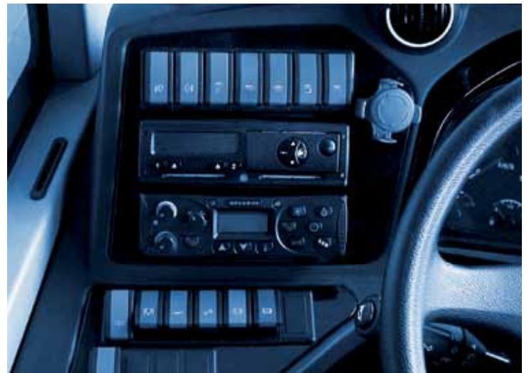
SDC coach: integrated controls in the driver's section.
